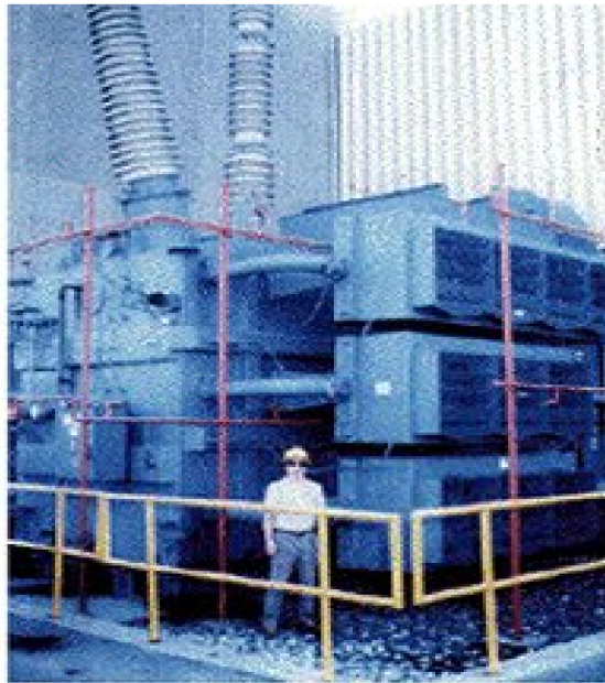
PJM Public Service Step Up Transformer
